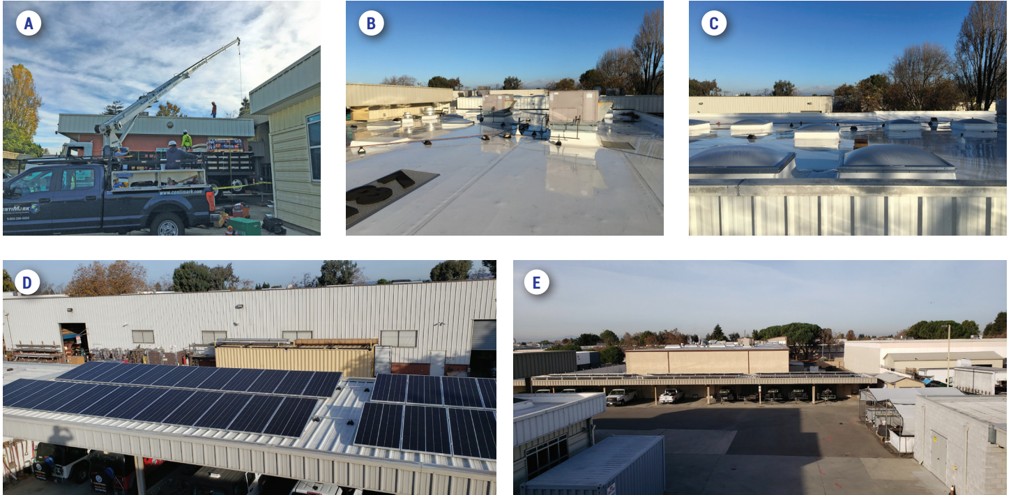
FIGURE 25: Roof replacement and solar panel addition. (A) Construction during the roof replacement. (B) Completed roof surface. (C) Newly installed skylights. (D) New solar panels on north parking rooftops. (E) New solar panels on west parking rooftops.
