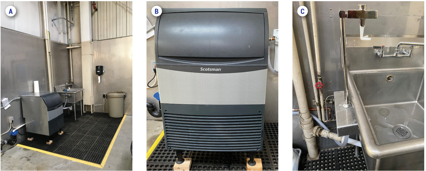
FIGURE 30: Shop improvements: (A) New ice and water filling station with stainless steel walls and ergo safety flooring. (B) New filtered ice machine. (C) New filtered water bottle filler.
