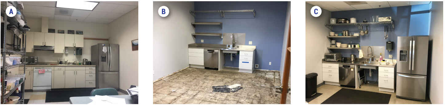
FIGURE 29: Kitchen/breakroom remodel. (A) Kitchen prior to remodel. (B) Kitchen during remodel. (C) Kitchen after remodel.
