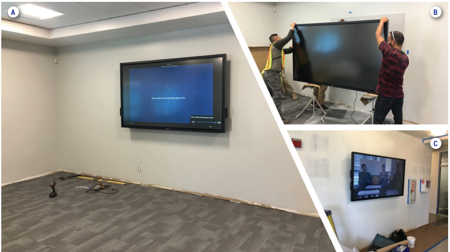
FIGURE 19: New touchscreen monitors. (A) Newly installed touchscreen monitor in the remodeled boardroom. (B) Installation of the new touchscreen monitor in the boardroom. (C) New touchscreen monitor at the front entry.
