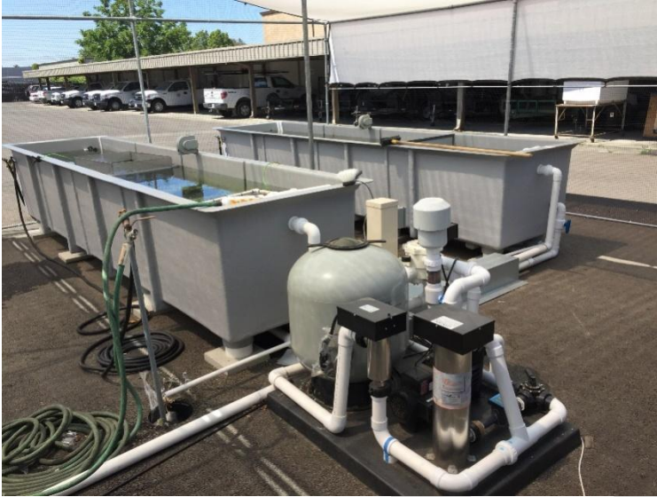
Two new tanks and pump system
